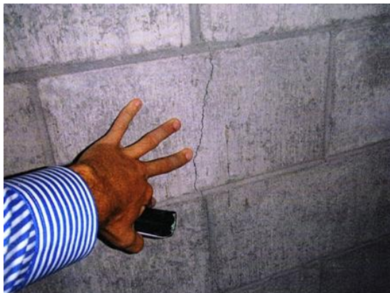
Damage from the Boxing Day earthquake at Lyttelton Church
