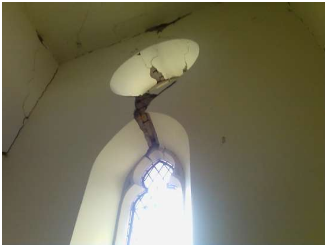
Damage Durham Street Methodist Church Tower
