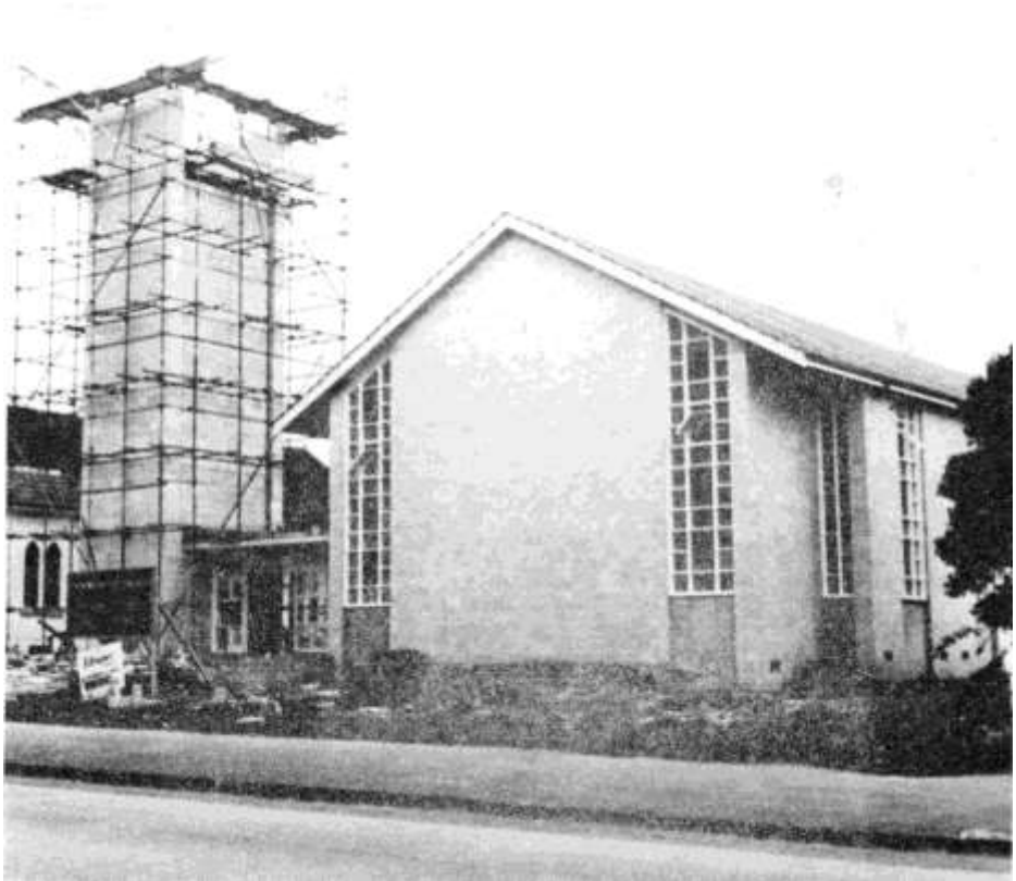
The Takapuna church being built in 1959. Vibrapac blocks by Winstone Ltd, photograph by Auckland Star.
