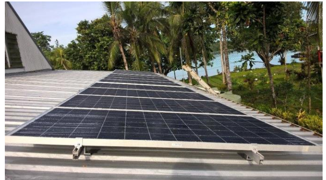
Solar Panels installed on the roof of the auditorium
