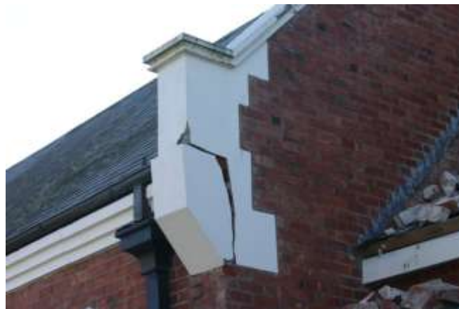
Damage to corner of Woodend Church
