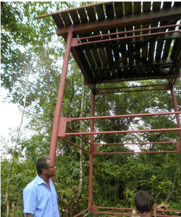
Brian Bird at the newly built tower for the storage tank to supply water from the borehole
